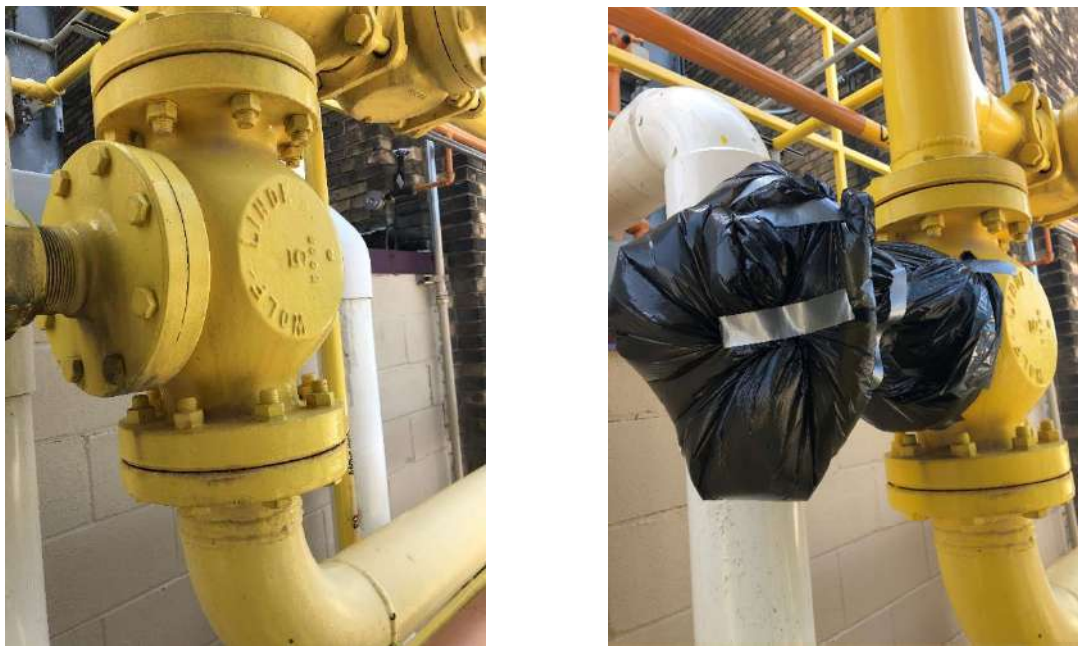
Figure 2. Shutoff valve on the high-pressure side of an ammonia refrigeration system (left) being bagged (right) to quantify refrigerant leakage from the bonnet gasket or stem packing.
