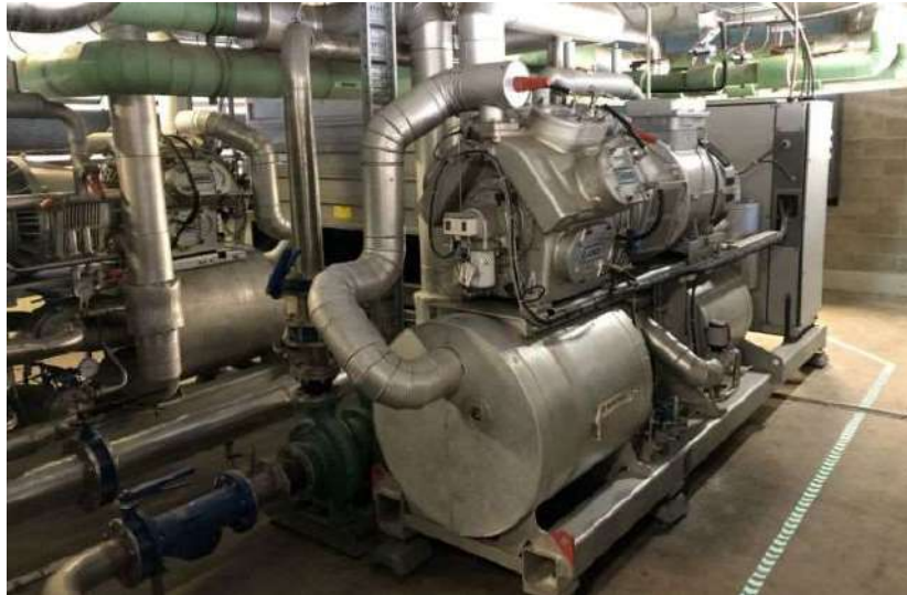
Figure 5: Pair of ammonia chillers cooling the Logan City Council administration building in Queensland, Australia (Courtesy: Scantec Refrigeration Technologies, Australia).
