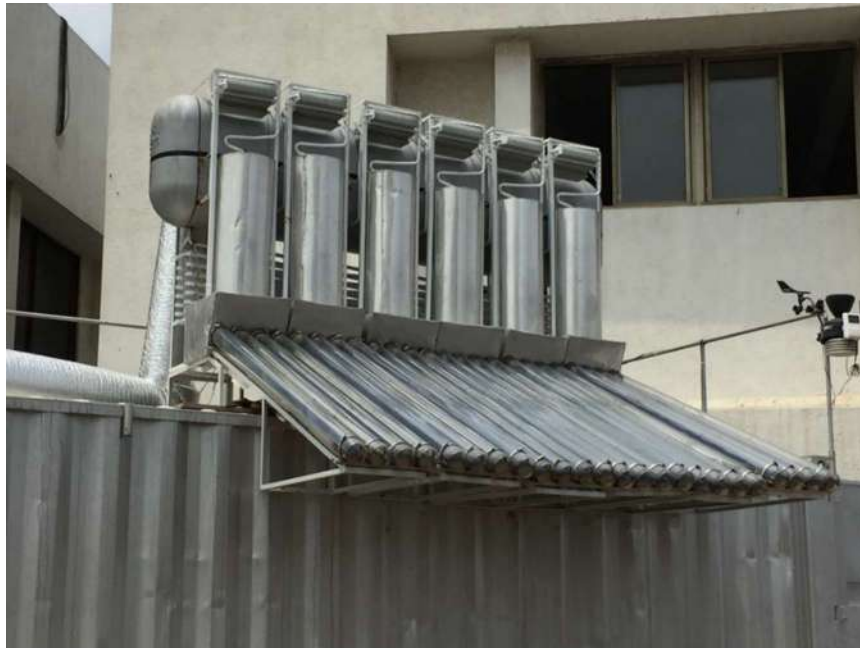
Figure 8. Ammonia-based diffusion absorption solar air-conditioning system under field trial in India (Courtesy: Solar-Polar, UK).
