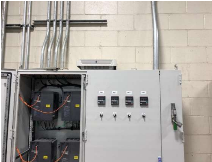
Figure 10. Example of several VFDs mounted in an enclosure. Notice the spacing between the VFDs and also the fan on top of the cabinet.
