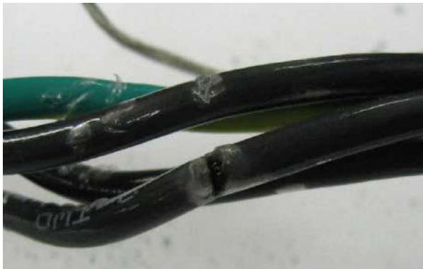
Figure 6. Example of cable pitting caused by corona discharge on THHN wire (source: Lutze 2019a).
