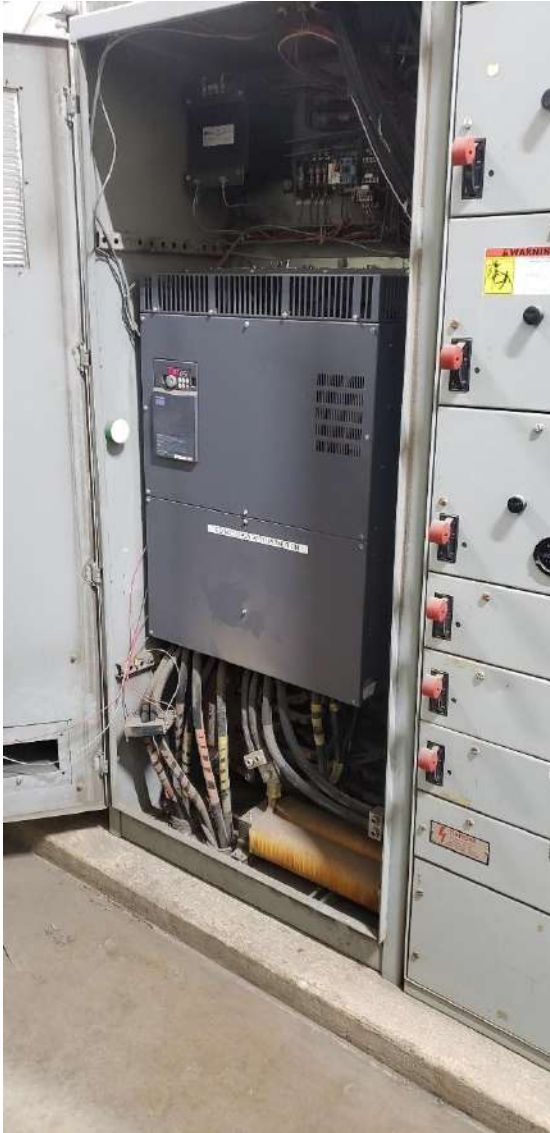
Figure 16. Example of a poorly maintained VFD. The end user found a defective fan on the VFD along with a fair amount of dirt and dust, which resulted in an overtemperature error.
