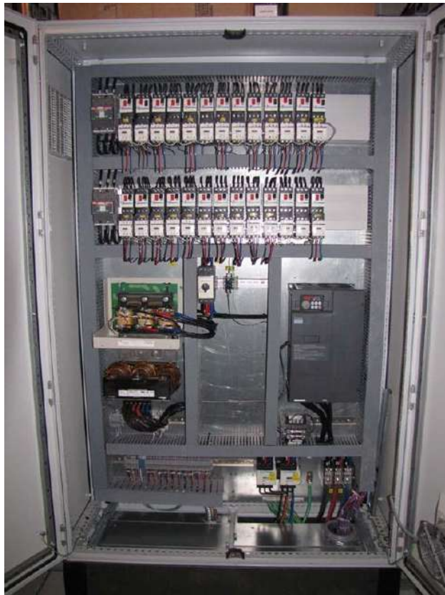
Figure 11. VFD mounted in a panel with other control devices. Note the depth of the cabinet and the spacing around the VFD.
