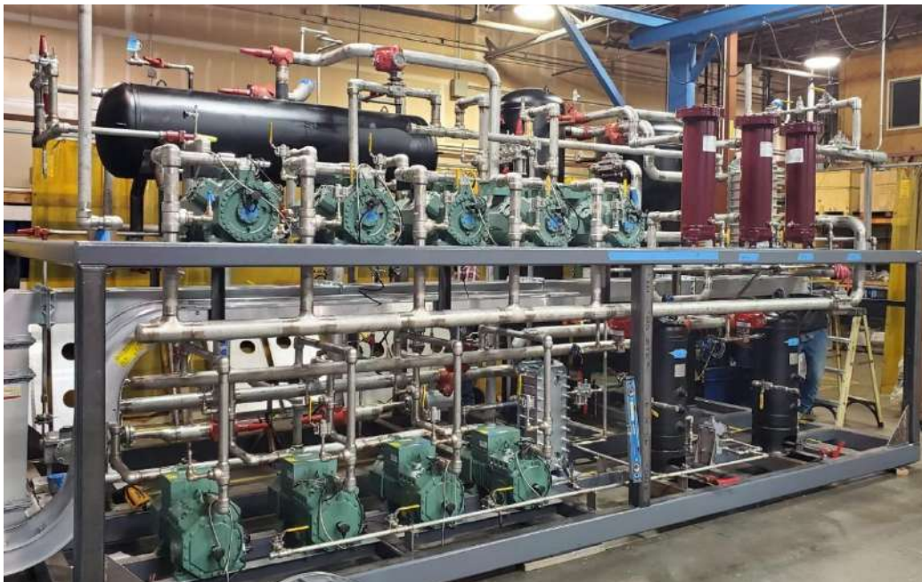
Figure 13. An industrial TC CO 2 refrigeration system 8 .
