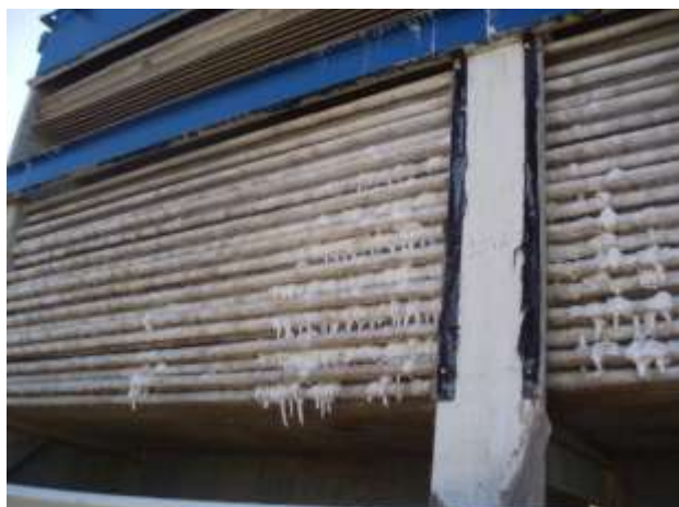
Figure 1. Consequences of poor condenser operation.
