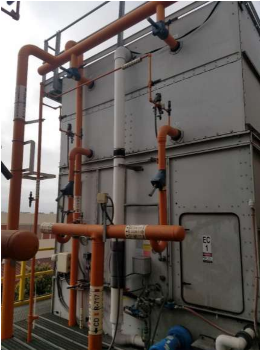
Figure 3. The “north” condenser (EC1) at the facility. The “south” condenser is off-frame to the left and is installed in a mirror fashion to EC1.
