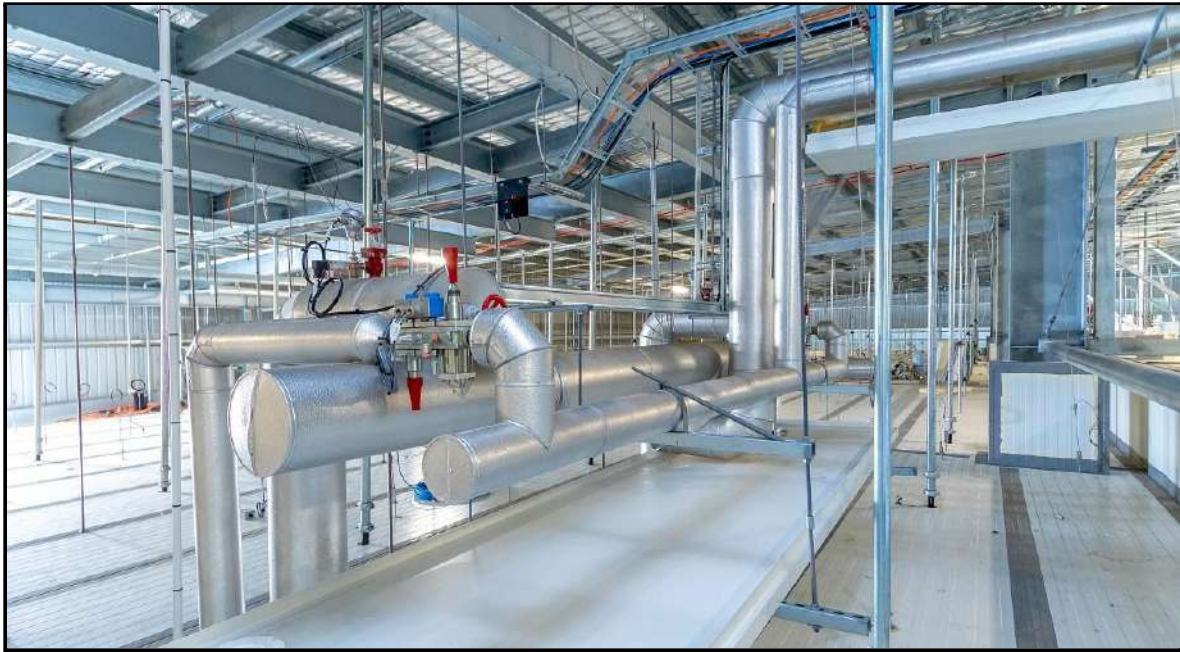
Figure 6. Ceiling cavity with typical suction risers between evaporators and main NH 3 pipelines.
