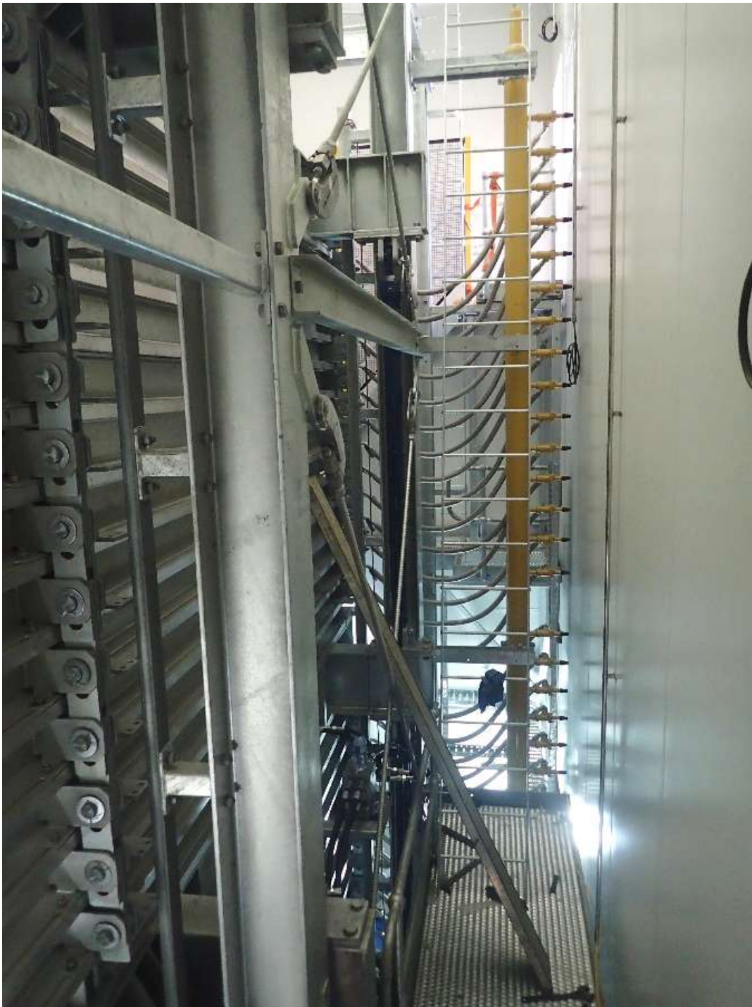
Figure 10. Installed plate freezer.
