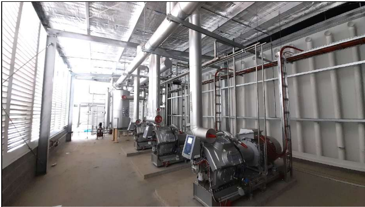
Figure 11. Centralized DX \text{NH}_3 refrigerating plant servicing small abattoir with blast freezers, freezer store, carcass chillers, and processing room in South Australia
