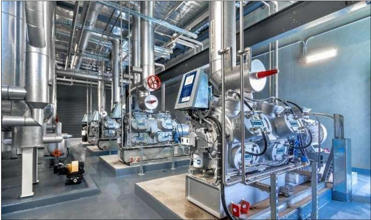
Figure 7. Low-charge NH 3 engine room.
