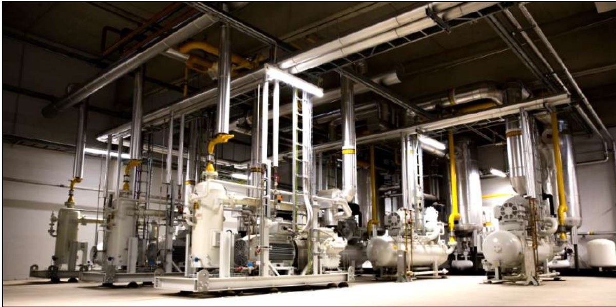
Figure 13. Centralized, low-charge -40°C (-40°F) DX NH 3 refrigerating plant, Hamburg, Germany.
