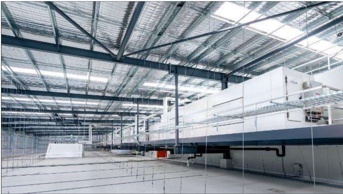
Figure 8. Insulated coolers in the ceiling cavity.
