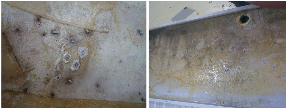
Figure 4. Corrosion damage observed in the drain tray.
