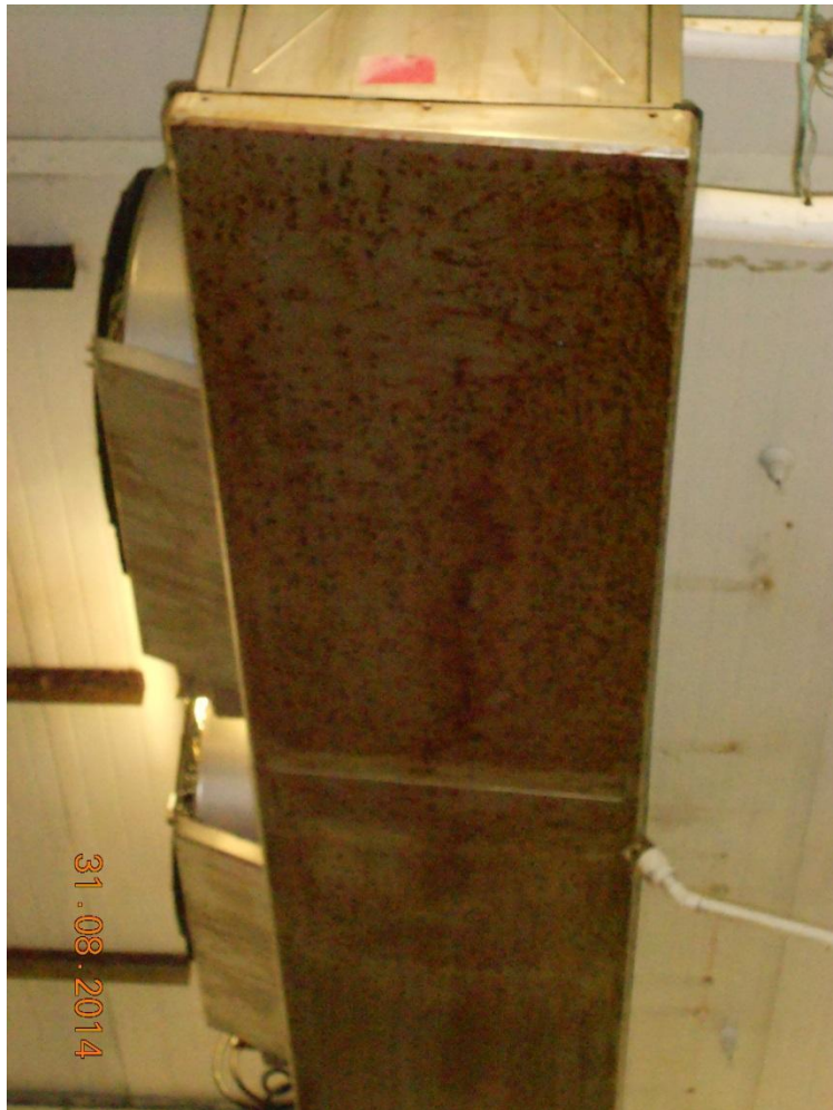
Figure 6. Corrosion observed on the drain tray surface.
