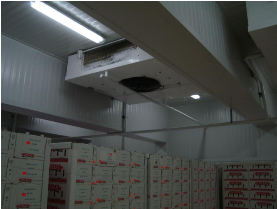
Figure 3. Location of the evaporator in the cold room.
