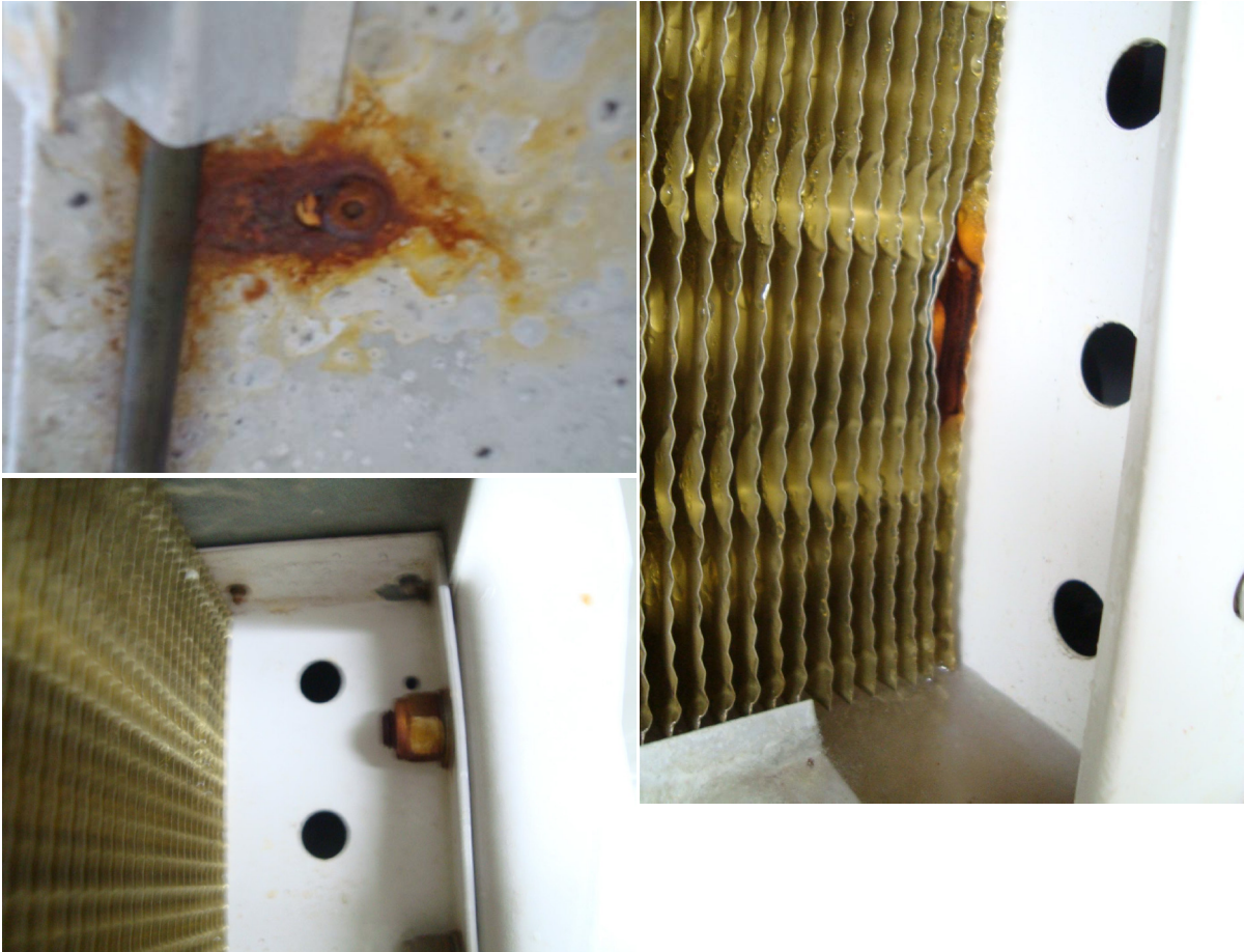
Figure 2. Corrosion on unit casings.
