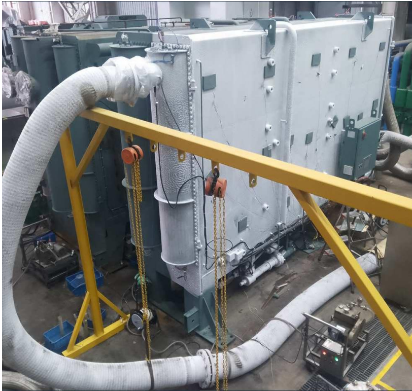
Figure 5. Single-effect two-stage absorption chiller producing 18°F (– 8°C) chilled water during testing.
