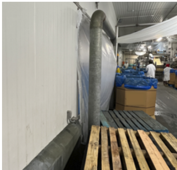
Figure 4: Example of incorrect air balance between process space (right) and construction zone (left).
